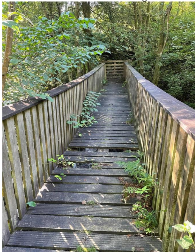
Footbridge currently closed due to safety concerns
